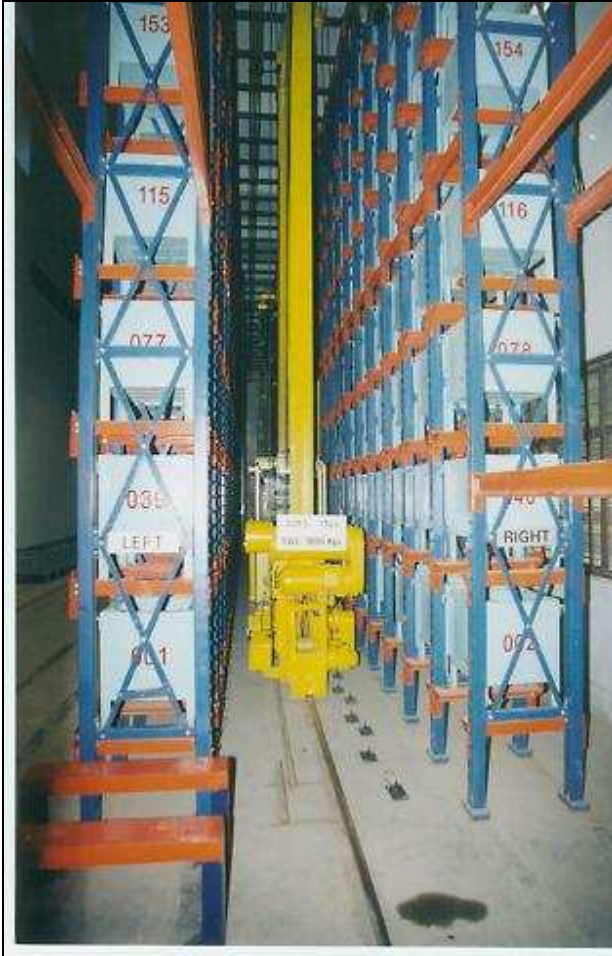
Figure 4: ASRS with crane and bins stored in racks
